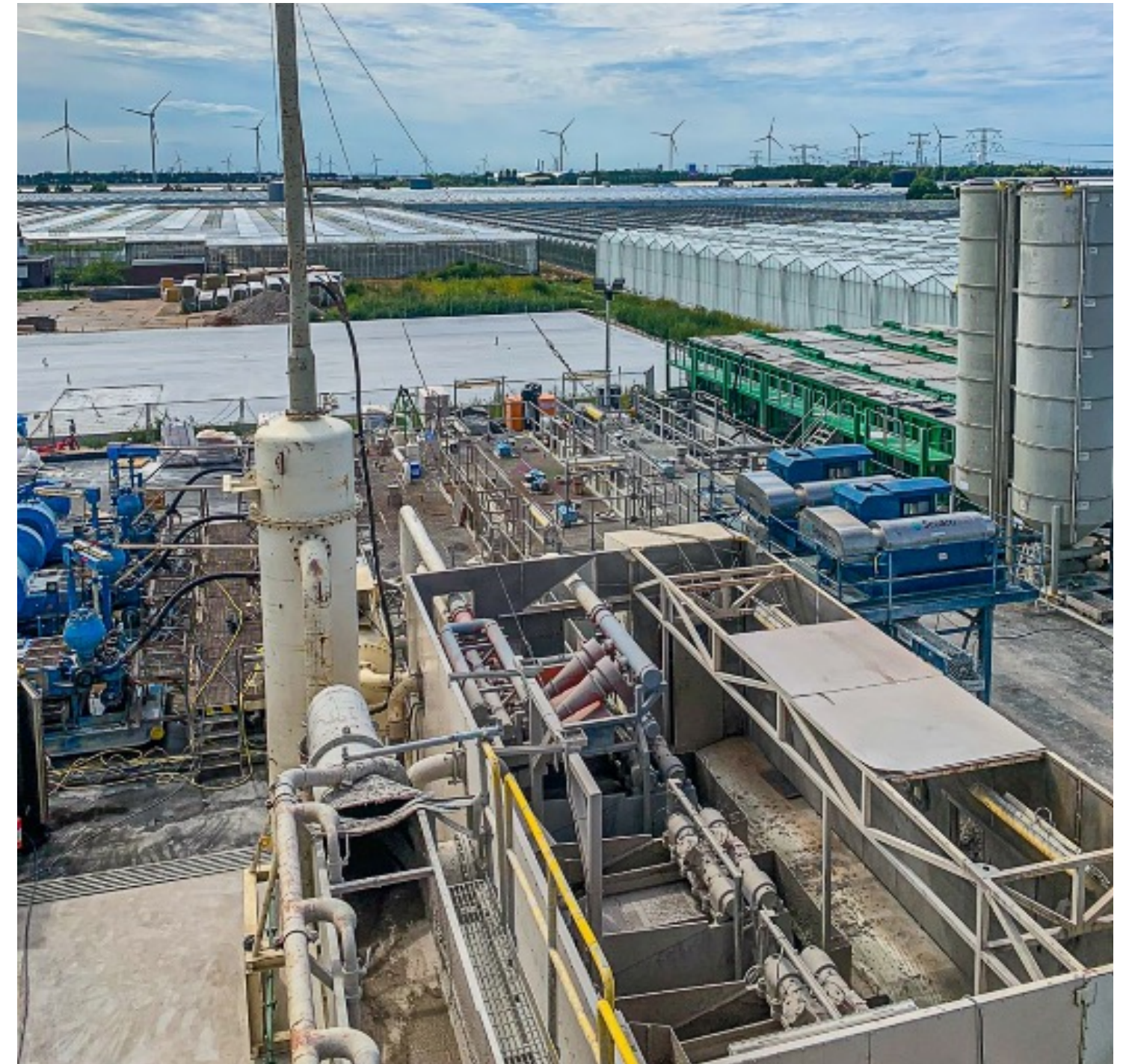
REF: View from Rig Floor of Geothermal Heating District Infrastructure
